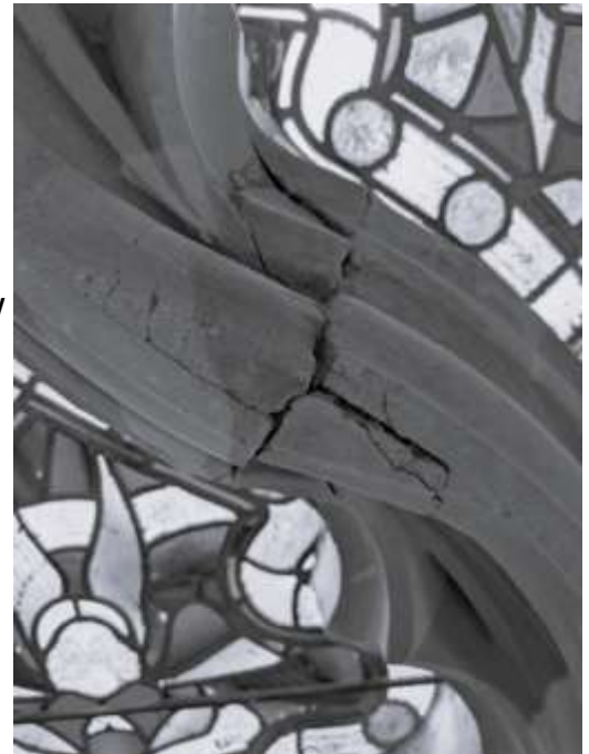
Example of a crack in one part of the tracery of the North Transept window.
